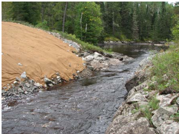
Stream bank rehabilitated using erosion control blanket and seeding at Beaver Creek Road bridge removal site.
