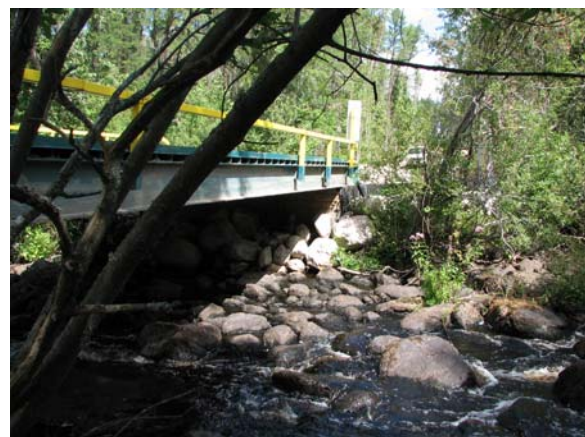
Effective Use of Erosion Control Material and Rip Rap on Portable Bridge Installation
